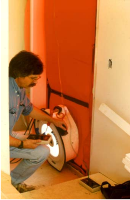
Photograph 7 – Portable Pressurization Fan
